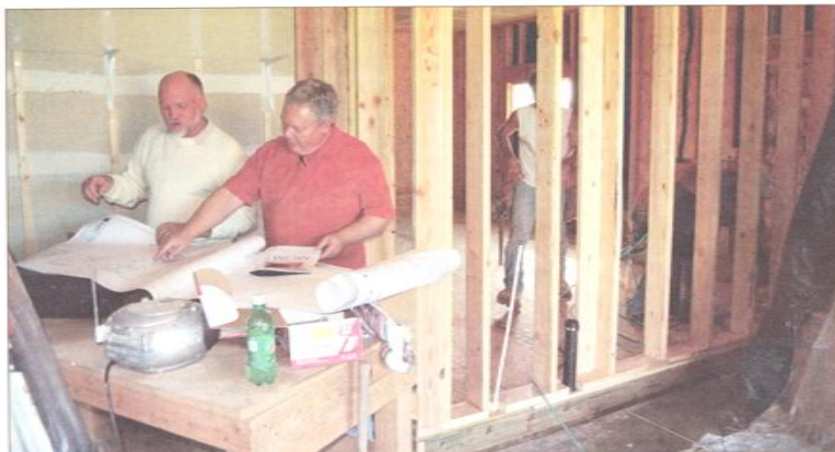
Aging in place specialist John Frazier (left) discusses remodeling plans with Eagle homeowner Joe Mortenson. Mortenson is remodeling part of his garage and home in order to better accommodate the accessibility needs of his elderly mother. Behind them, contractor Brett Roth of Roth Construction, Boise, and carpenter's helper Gabe frame a new bedroom wall.
